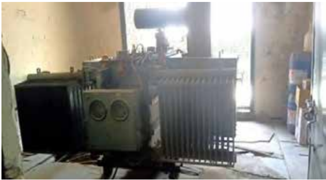
750 KVA Transformer at ESS-5
