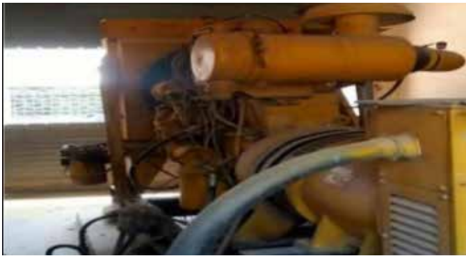
125 KVA DG Set at ESS-5
