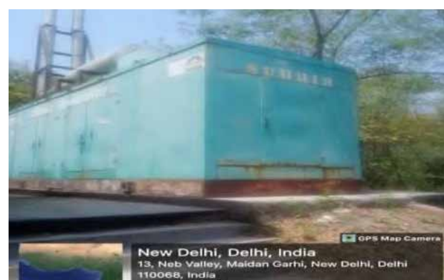
DG set 750KVA at ESS – 1
