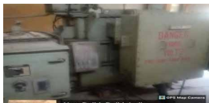
Transformer at ESS-1
