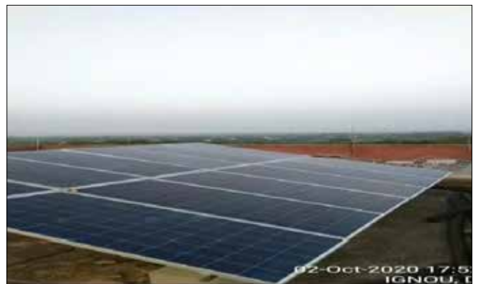
Block No.-15 Rooftop Solar Plant
