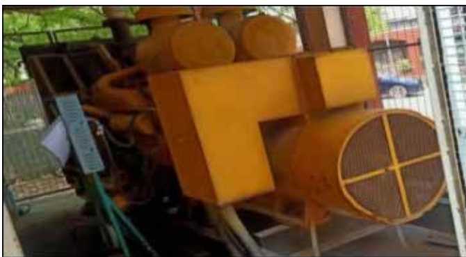
437.5 KVA DG Set at ESS-5
