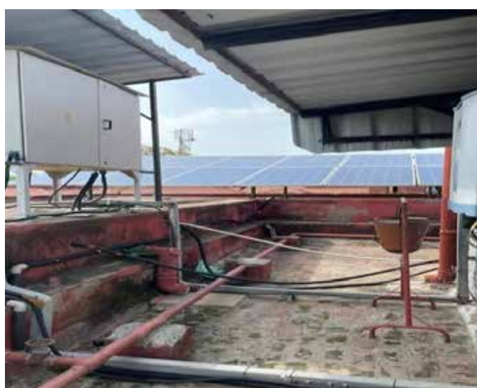
Solar Rooftop System at Academic Block 3
