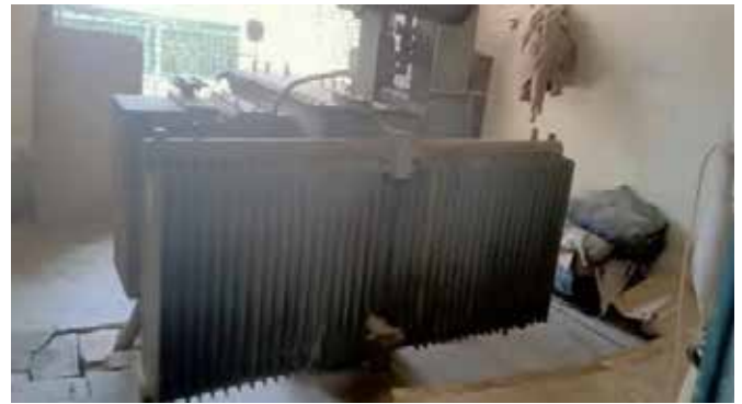
1000KVA Transformer at ESS-5
