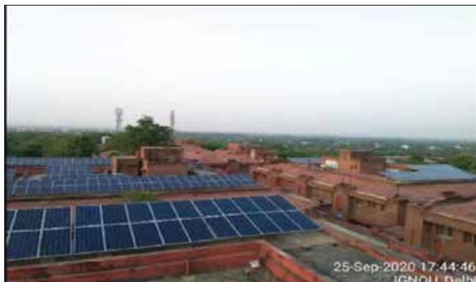
Rooftop Solar Plant at Different Academic Blocks
