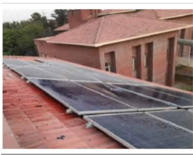
EMPC Roof Top Solar Plant
