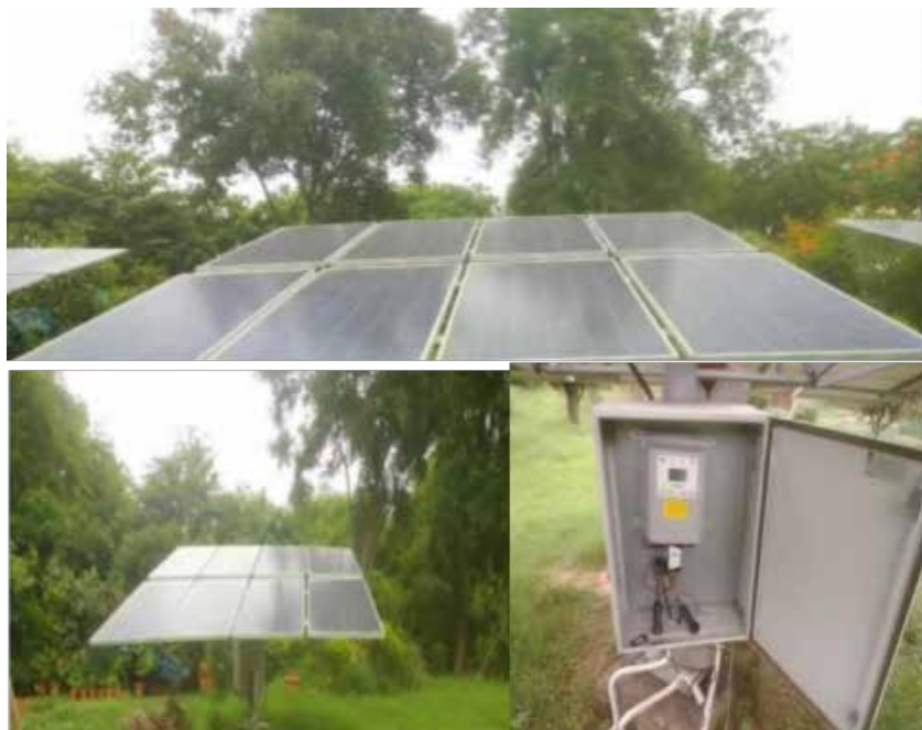
Solar Water Pumping System at IGNOU
