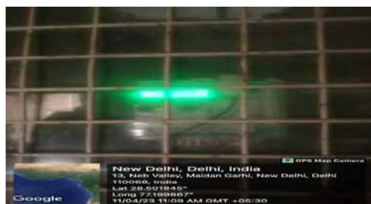
HT Net metering of BSES Sub Station
